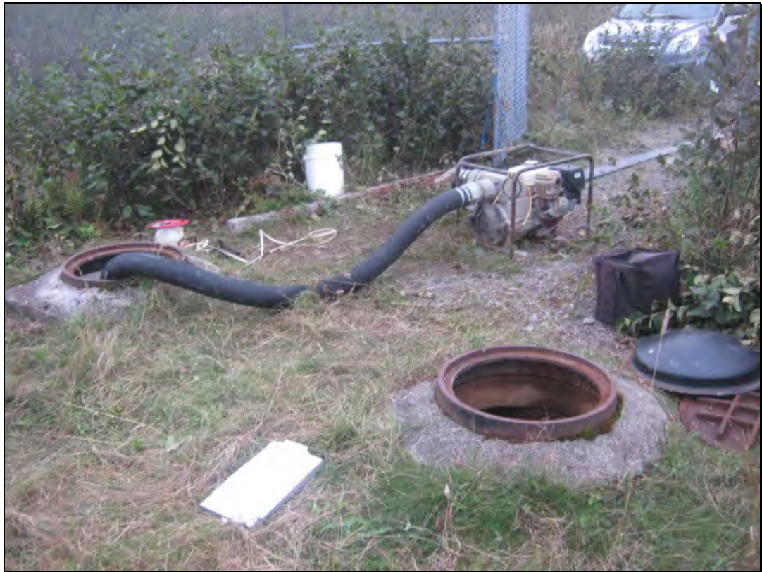
Photo 9: View, looking southwest, while pumping leachate from the PLCS and SPCS valve chambers in October 2013.
