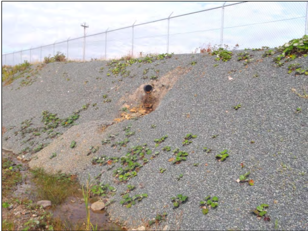
Photo 7: View, looking northeast, of the groundwater interception drainage system during the August 2013 Site visit. Note discharge pipe without a rodent screen and iron oxide staining.
