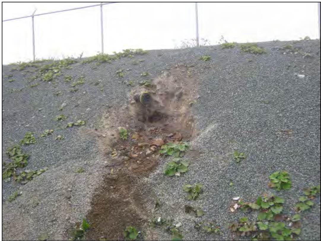
Photo 8: View, looking northeast, of groundwater drainage system discharge location with new rodent screen installed during the October 2013 Site visit.
