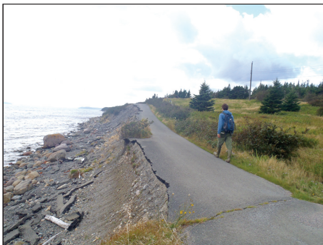
Plate 1. Coastal erosion is occurring along this road in O'Donnells, Avalon Peninsula. Ground- and surface-water flow are causing the sand and gravel to wash down the bank. During high tides, waves impact the base and wash the sediment away from the base of the slope.
