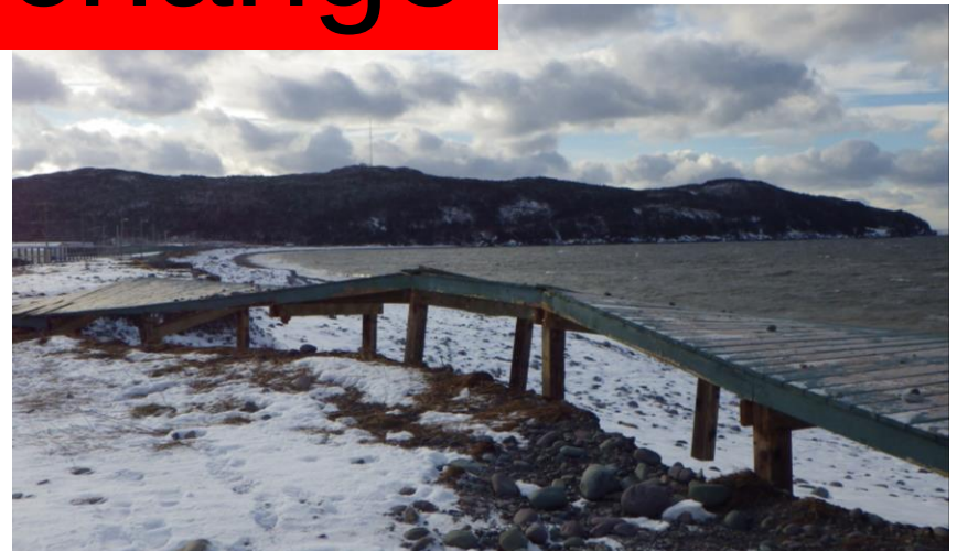
Storm surge damage, Placentia
